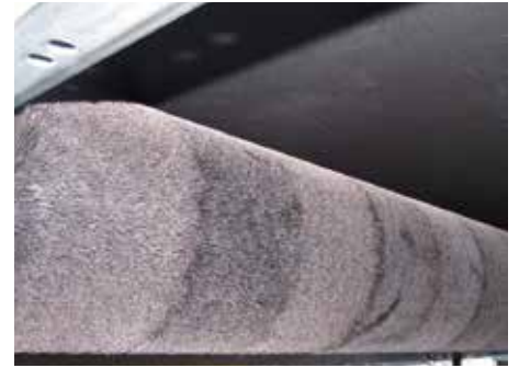
Belt cleaning equipment
